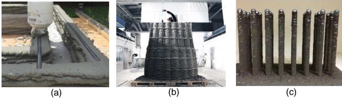
Figure 2. Reinforcement strategies using steel bars: a) placement of straight reinforcement bars in the print plane [8]; b) placement of reinforcement in horizontal as well as in vertical direction [9]; c) 3D-printed reinforcement bars using WAAM welding process [10].
